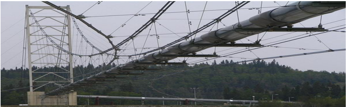
Figure 19 Example of a Pipeline Bridge
